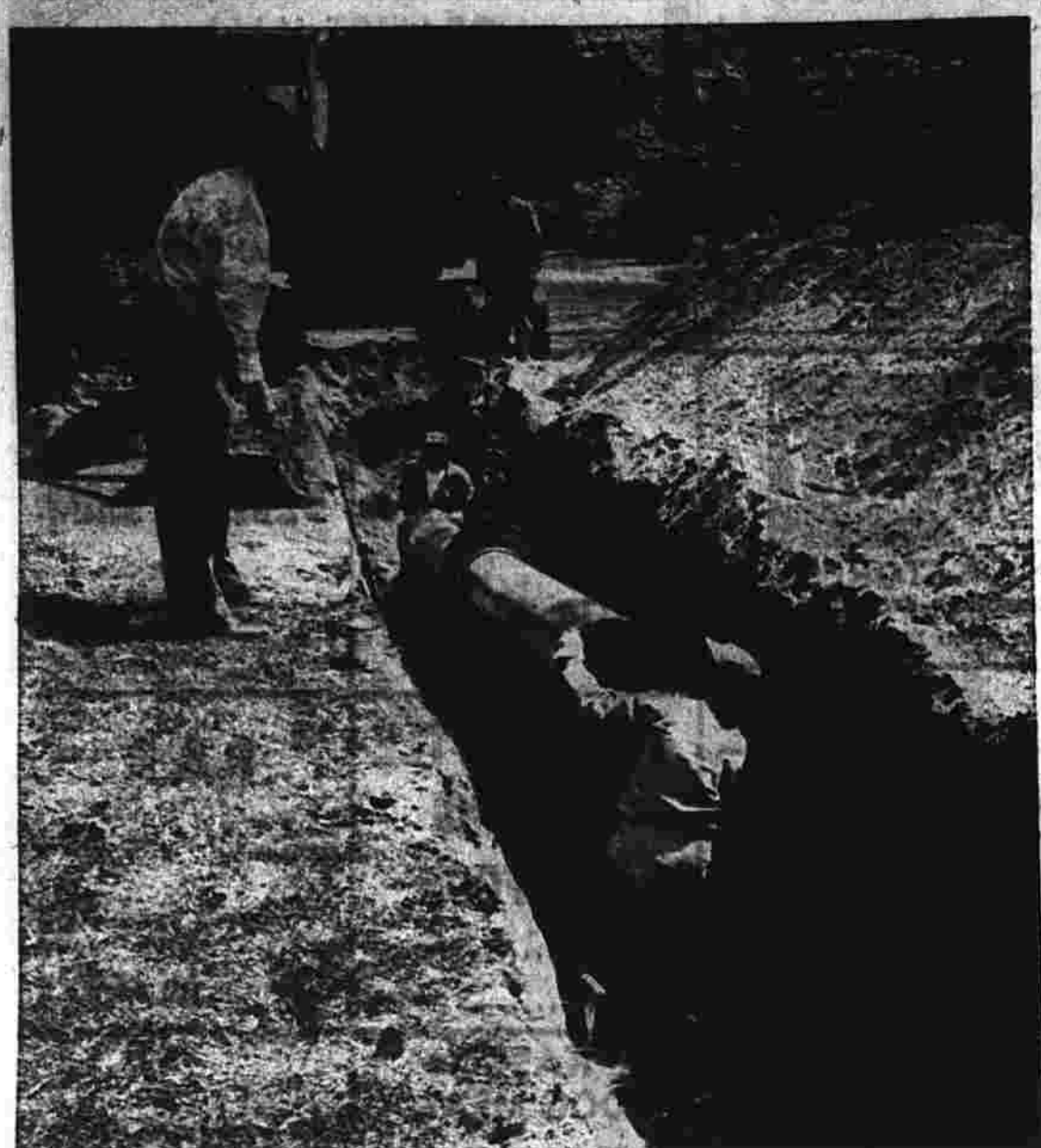
Workers make a 16-foot section of 12-inch pipe in Hilliard St. part of a new main being installed by the Manchester Water Co. to supply North End residents with well water.
